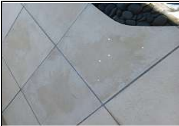
Wrong Application of Sealer
