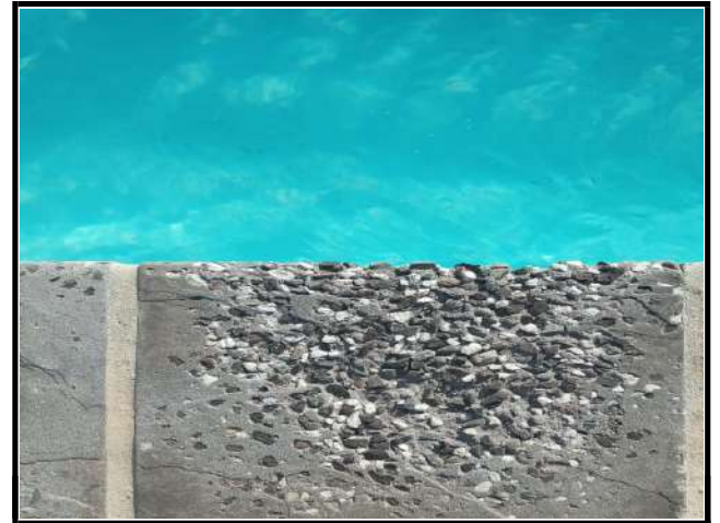
Product not Sealed (Salt water damage)
